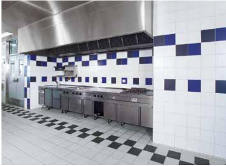
Easy cleaning in kitchens Dempsey Barracks, Paderborn, Germany / Architect: BLB NRW, Ms Lachmann / Photo: Fotostudio Bieleesch
